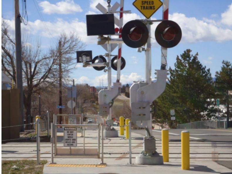
Figure 8 Pedestrian Crossing with Swing Gates
