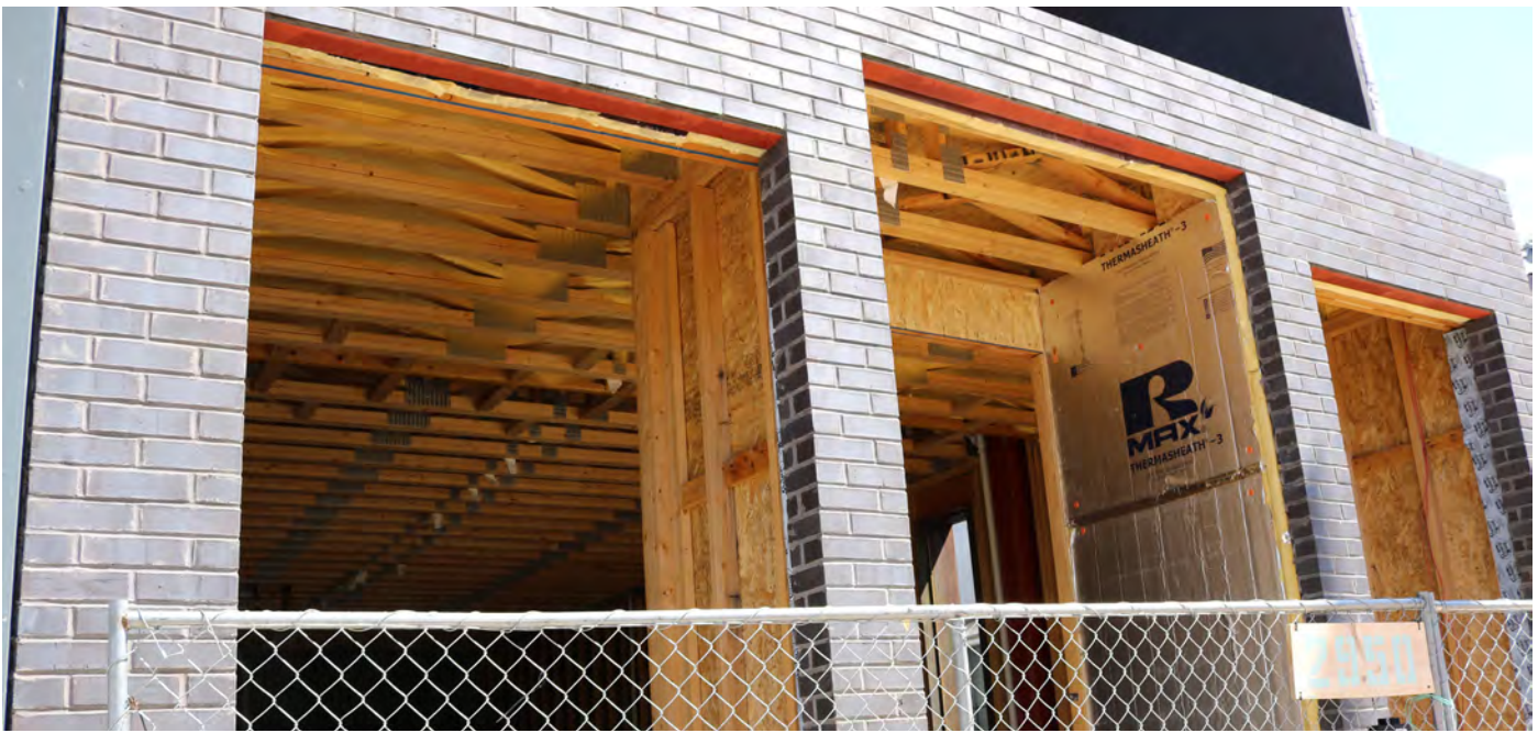
Small scale infill construction in the 2900 block of Welton Street on a previously vacant lot.
