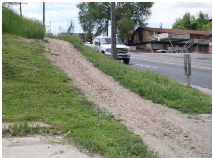
There are many problems with the existing condition of Sheridan Boulevard including poor pedestrian conditions.
