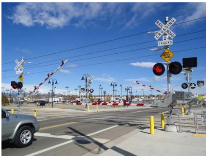
FIGURE 7 - QUAD GATES / DELAYED GATE ARM CLOSURE
