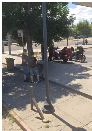
Figure 3-34: Poles Obstructing Path of Travel at Lipan St & W 38th Ave in Denver (14991)
